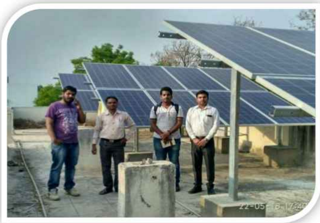
10 KW project Jain Solar at Girls Hostel
